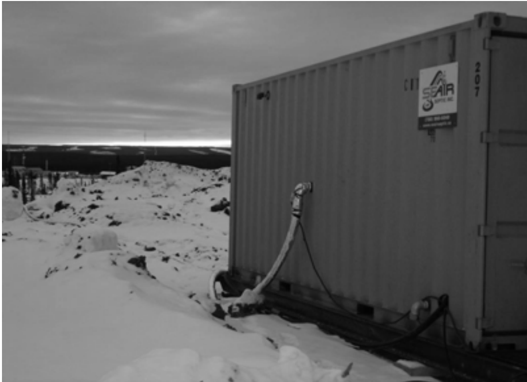
Picture 1: Seair Portable Wastewater Treatment Plant
