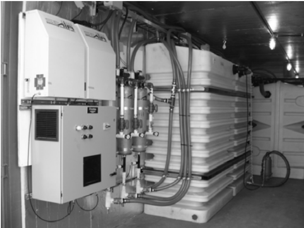
Picture 2 : Inside of PWW40 Treatment Plant
