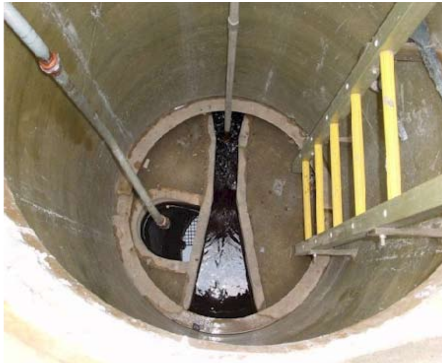
A Parshall Flume installed in a pre-fabricated manhole. Note the ultrasonic transducer over the stilling well on the left.
